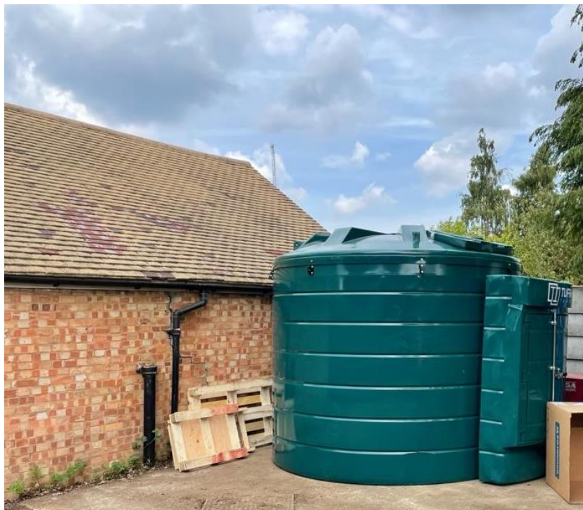
Fig.4 Photograph of fuel tank in situ (source: applicant)
